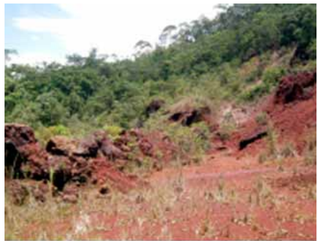
Figure 7 - Excavation in canga at the foothills of the Serra da Piedade; canga is used for road construction. Photo: M.M.M.Machado
